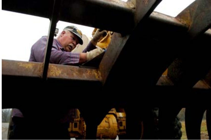
Milbocker & Sons Contractors road foreman Ron Rantz, of Jenison, installs a brush rake on a front end loader Monday. "We're just getting started," Rantz said of the work. Work on the bridge is expected to be finished by Nov. 15, 2008.
